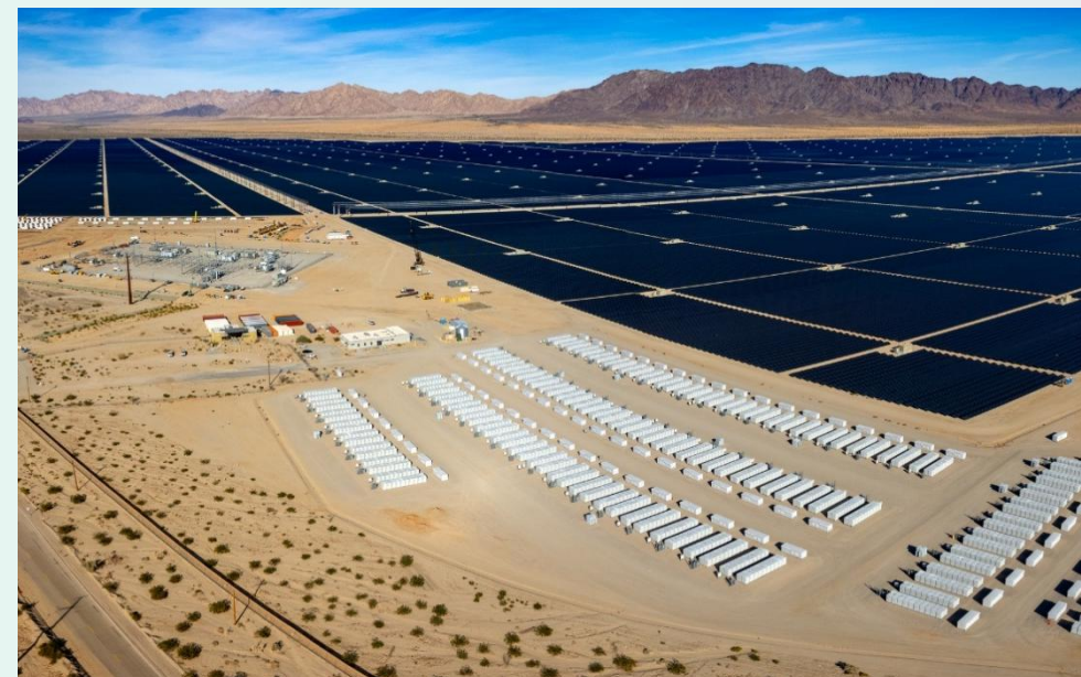
The Centennial Flats project is located in Arizona, US, and was Eolus's first sale of a combined solar and battery project. It comprises 500 MW of solar power and 267 MW of battery storage. The project was sold in 2022 and is expected to reach full commercial operation during 2026.
